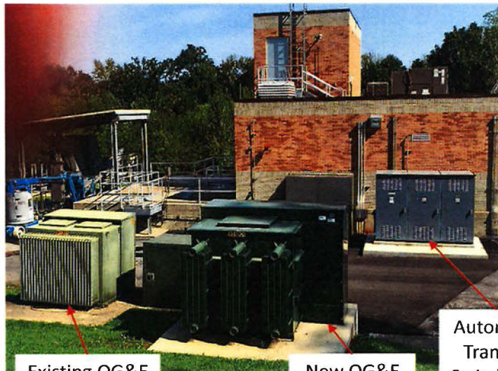
Existing OG&E Transformer
