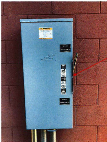
Manual Transfer Switch
