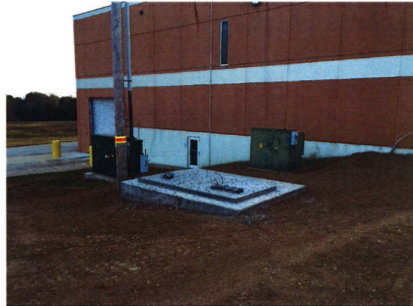
Building C – Equipment Pad
