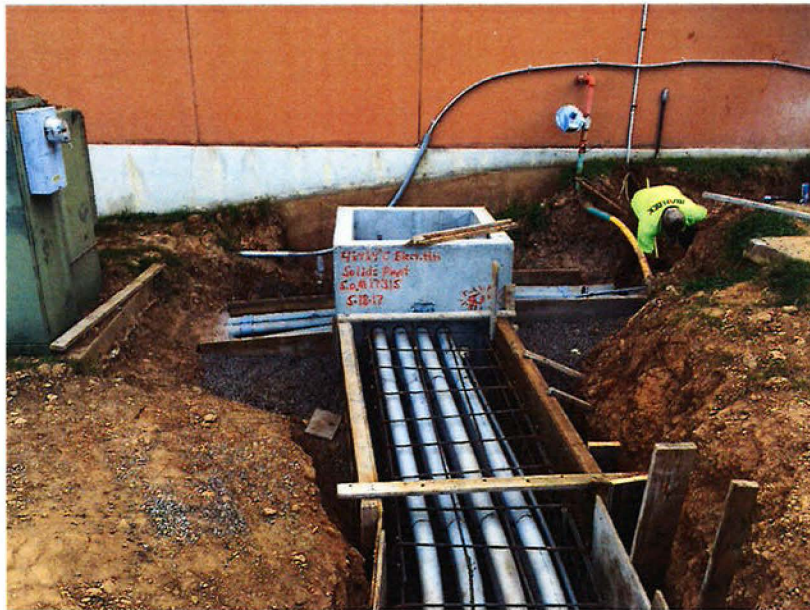
Building C – Conduit Runs
