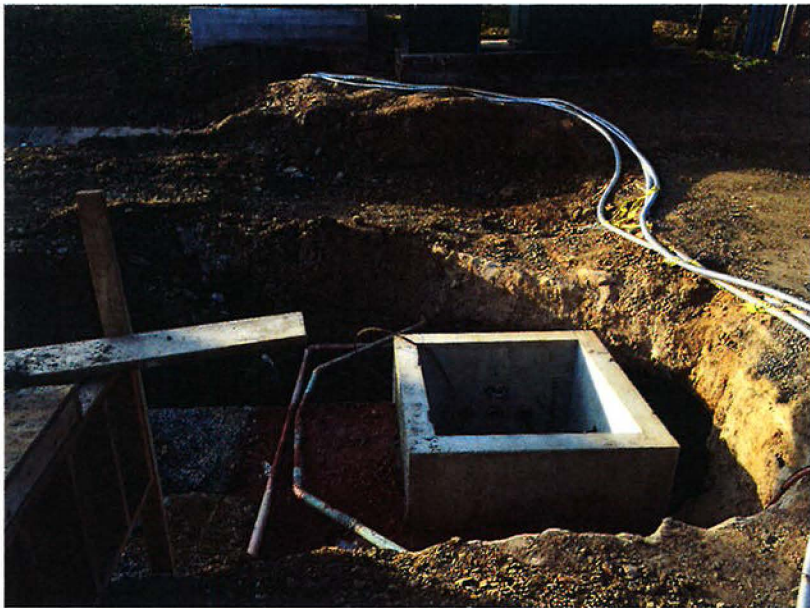
Building I – Junction Box
