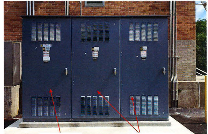
Controls & Meter Section
