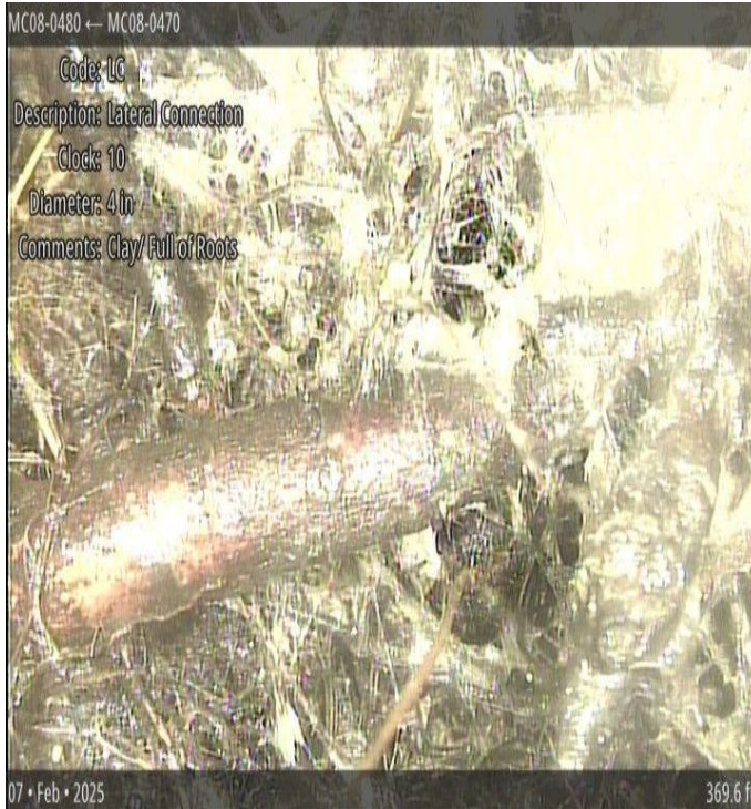
PRE-CCTV VIDEO INSPECTION OF SANITARY SEWER MAIN (ROOT INTRUSION OBSERVED)
